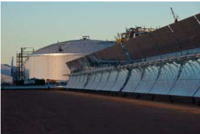
Thermal energy storage tank
