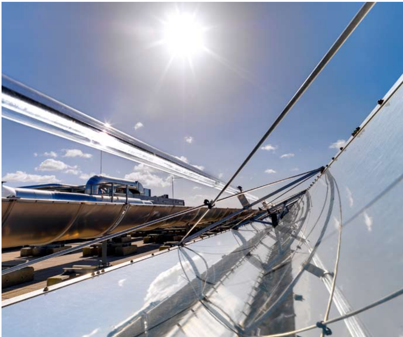
Parabolic troughs at an Abengoa solar plant
