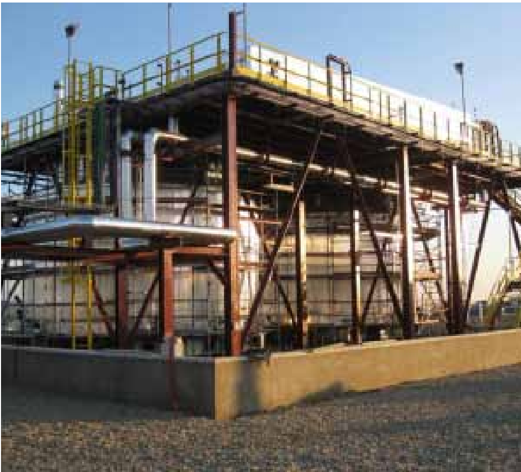
Molten salt storage pilot plant, operational since 2009 at the Solucar platform, Seville
