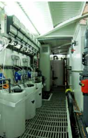
Seawater pretreatment pilot plant using membranes
