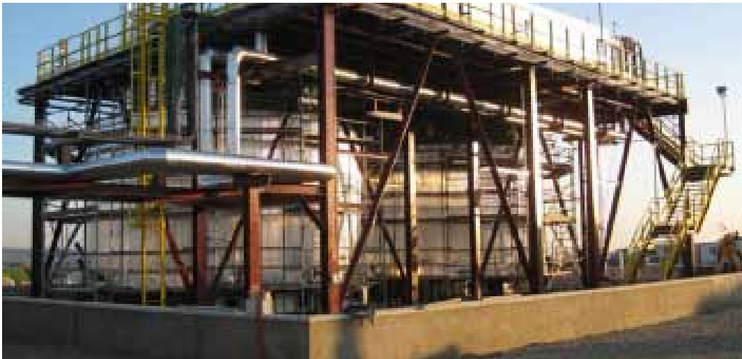
Pilot molten salts storage plant in operation since 2009 at the Solúcar complex, Seville
