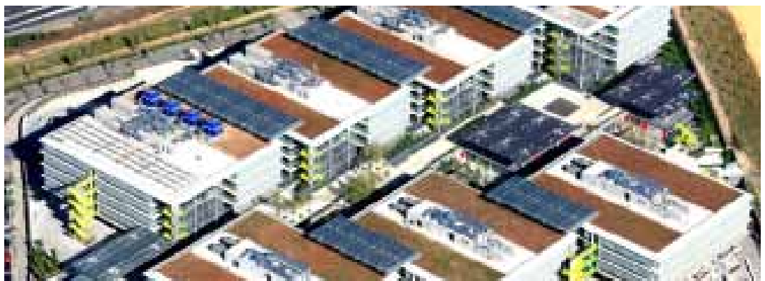
Industrial solar thermal facility for the climate control system at the Palmas Altas Campus
