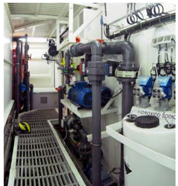
Befesa Water. Advanced pre-treatment systems pilot plant.
