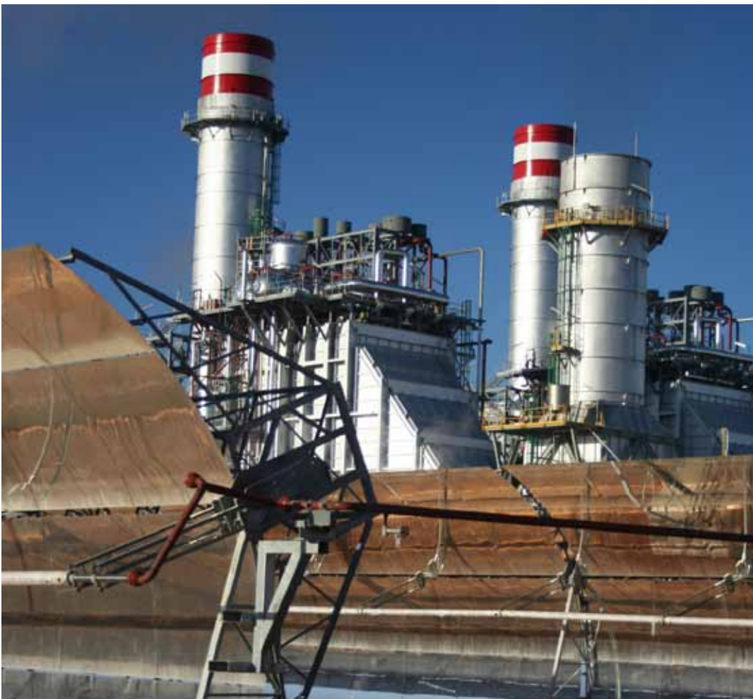
482 MW Ain Beni Mathar ISCC plant in Morocco
