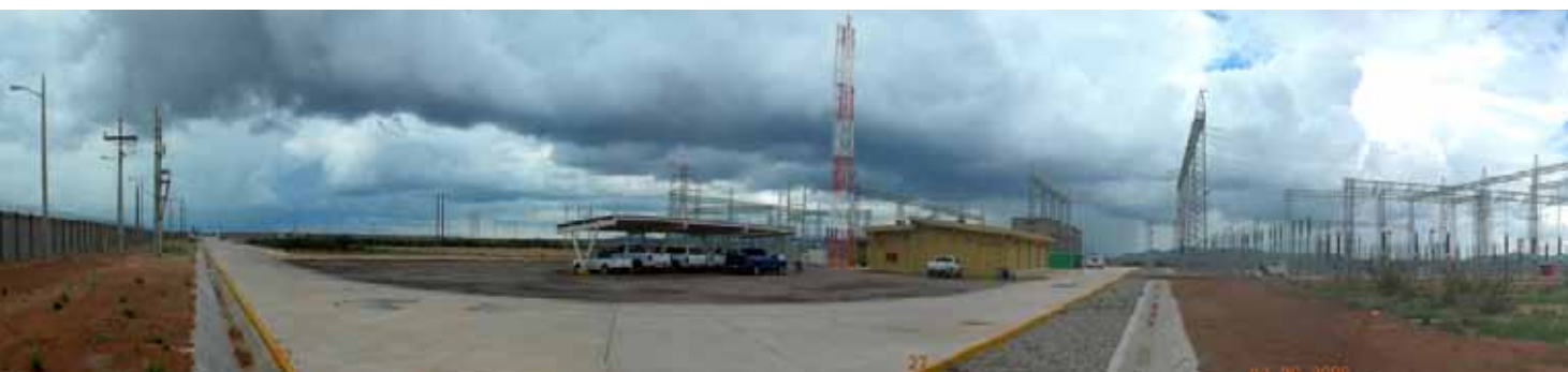
Mesteñas substation in the state of Chihuahua, Mexico
