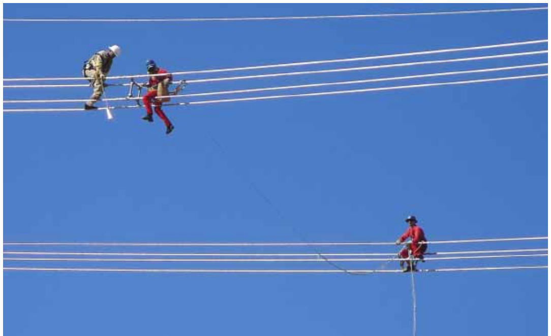
Abengoa Brasil employees carrying out O&M work on a power transmission line
