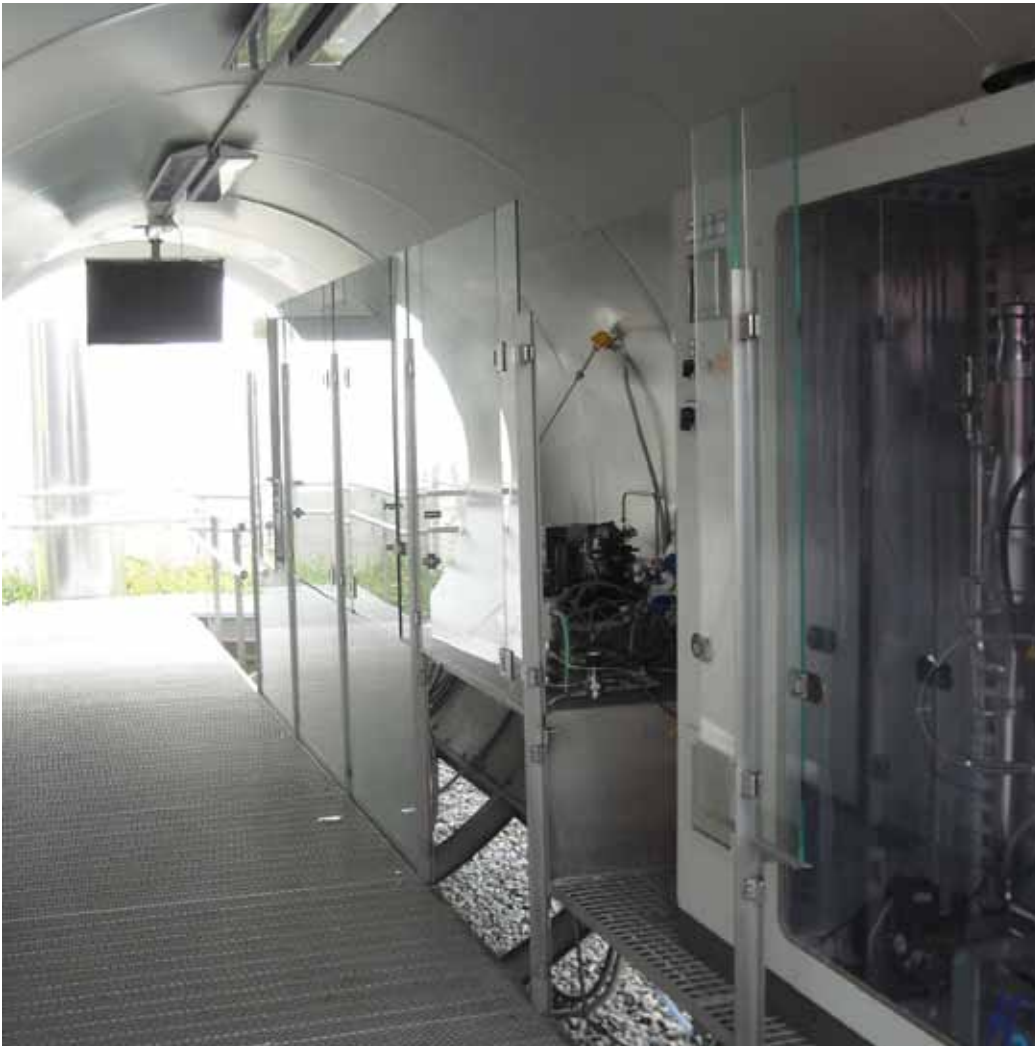
Hydrogen generation system and fuel cell for the Palmas Altas Campus
