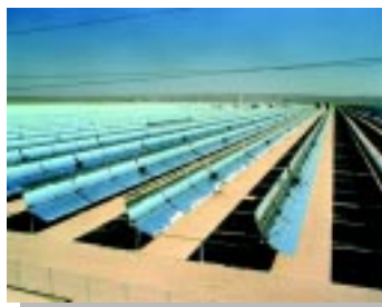
Solar thermal parabolic collector
